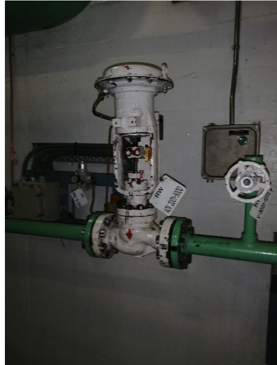
Figure 18. Liquid waste discharge shut-off valve
