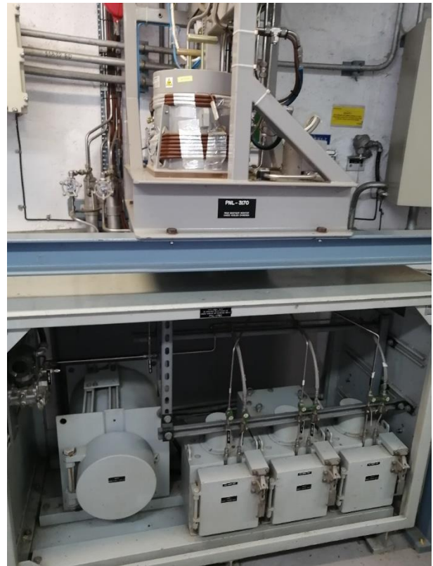
Figure 12. Garoña NPP stack emergency discharge monitoring system
