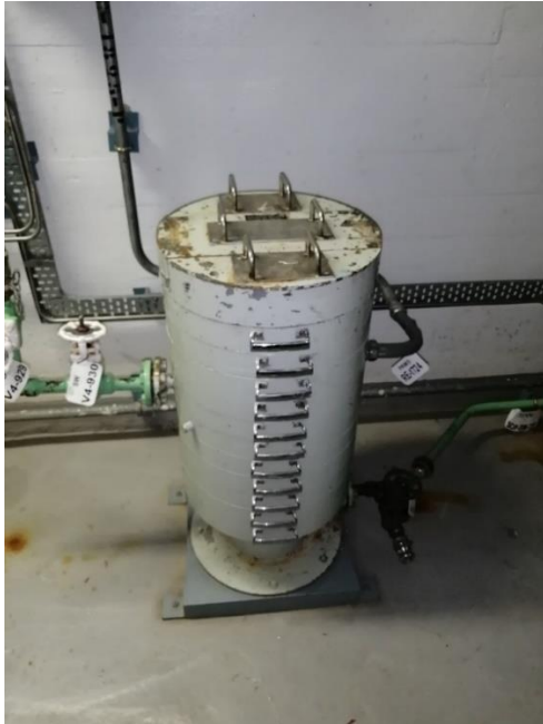
Figure 16. Service water discharge radioactivity monitor
