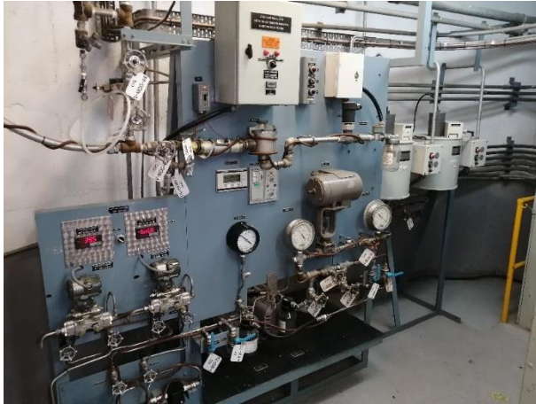
Figure 11. Garoña NPP stack routine gaseous discharge monitoring system
