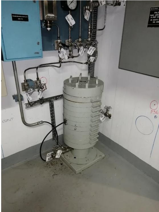
Figure 17. Liquid waste discharge monitor
