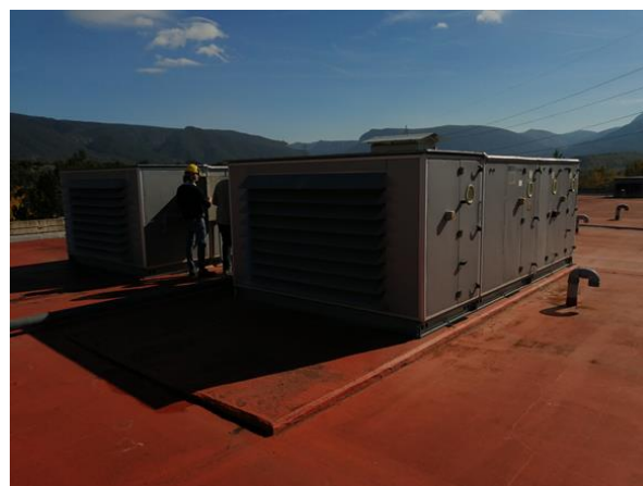
Figure 15. HEPA filters on the waste treatment building roof
